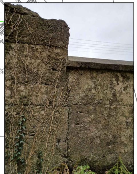
2 - VERTICAL AND HORIZONTAL CRACKING AT CONSTRUCTION JOINTS THROUGHOUT. APPEARS TO BE POOR QUALITY OF CONCRETE (I.E. SITE MIX CONCRETE AND ABSENCE OF REINFORCEMENT)
