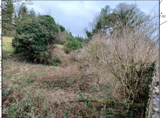
10 - NO ACCESS TO RANDOM RUBBLE STONE WALL AT LOWER SIDE DUE TO VEGETATION.
