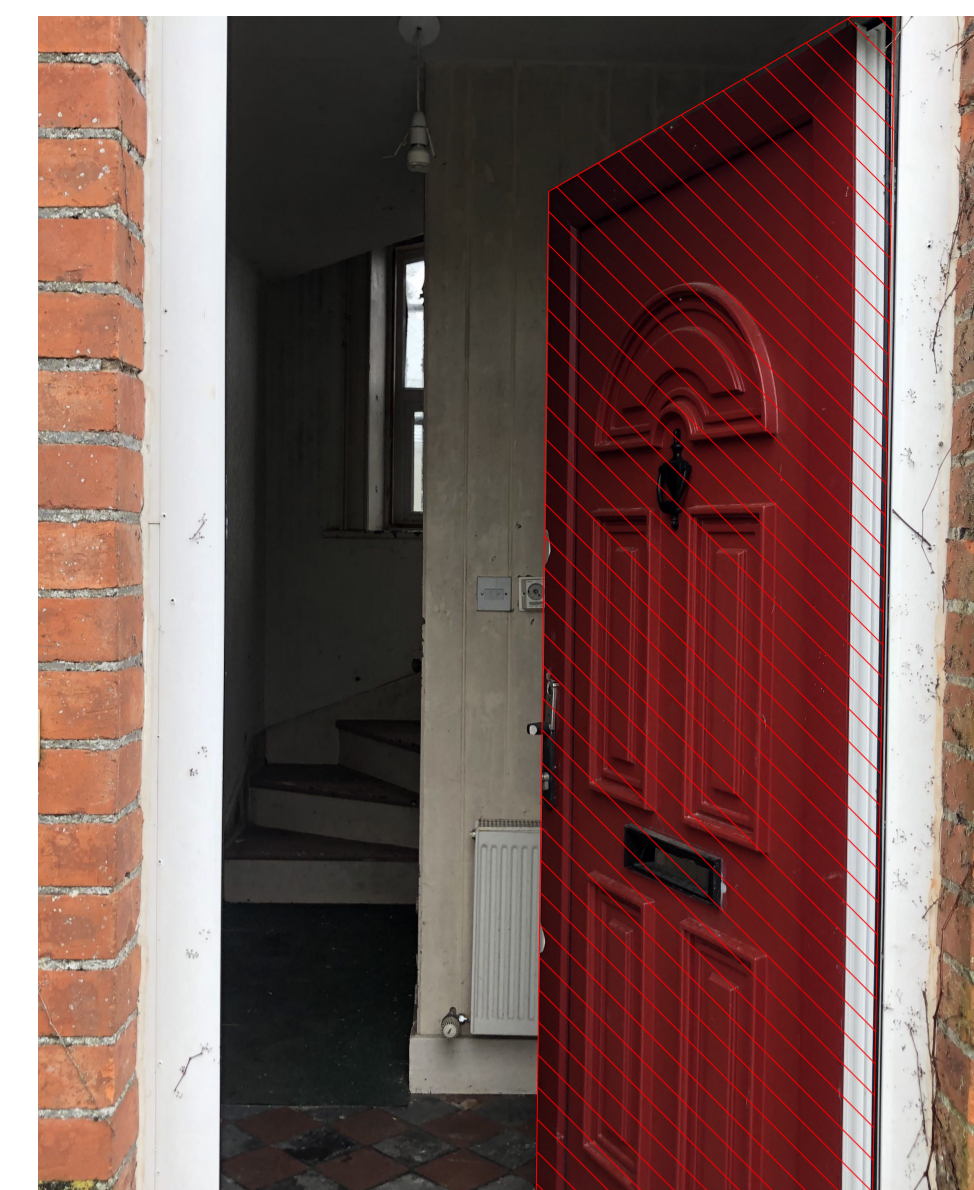
EXISTING PVC FRONT DOOR TO BE REPLACED
