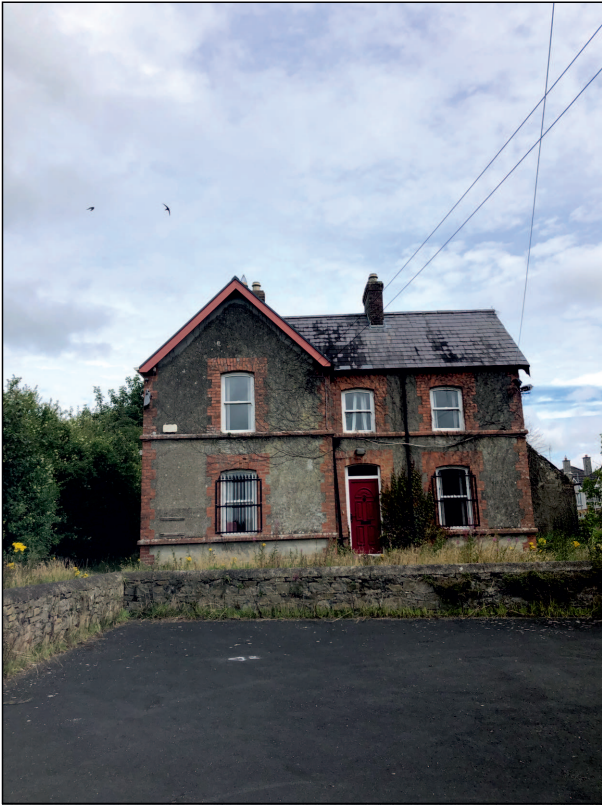
Plate 1: View of Old School Masters House facing the front building elevation in 2020
