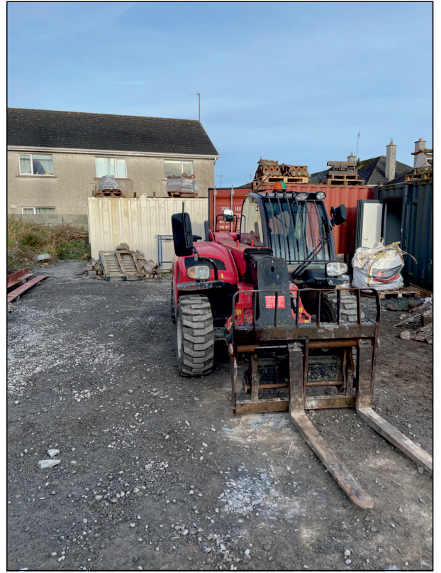
Plate 6: View of compound area to rear boundary wall of Old School Masters House
