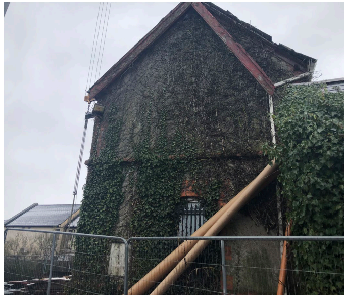
Fig 17: Elevation D. Evidence of climbing plants on side facade. Existing fascia board has been damaged. *Note picture was taken in March 2024 during works to former school-house.
