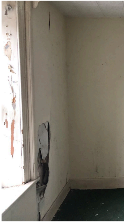
Fig 32: Internal Elevation 2.C. Wall has been damaged.
