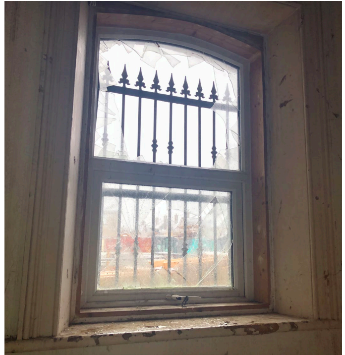
Fig 25: Internal Elevation 1.A. Window to staircase. Sash Window has been damaged.
