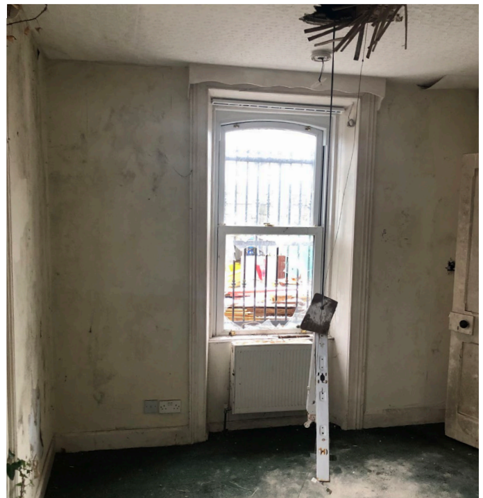
Fig 50: Internal Elevation 4.C. Sash Window has been damaged.
