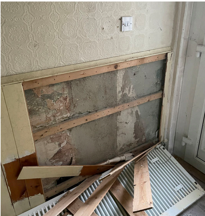
Fig 38: Internal Elevation 3.A. Timber dado panelling and existing radiator have been damaged.
