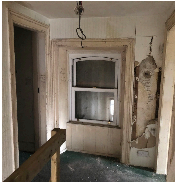
Fig 64: Internal Elevation 7.C. Existing window boarded up. Damaged plasterboard.
