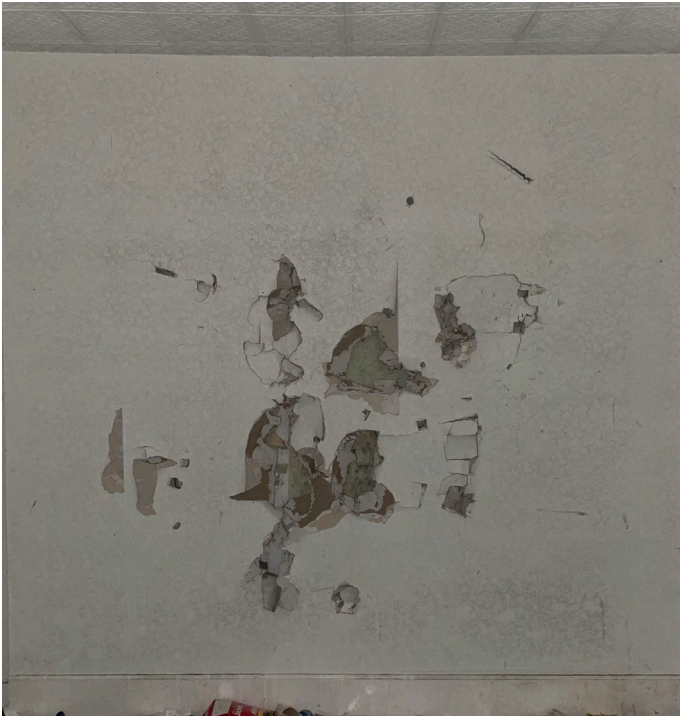
Fig 77: Internal Elevation 12.A. Plasterboard damaged.
