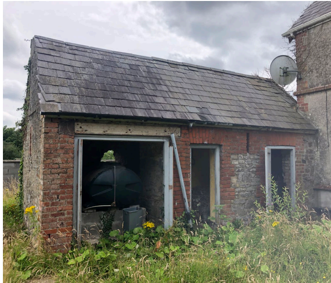
Fig 6: Elevation B. Stone/brick extension to rear of existing Master's House. *Note picture was taken in July 2020.
