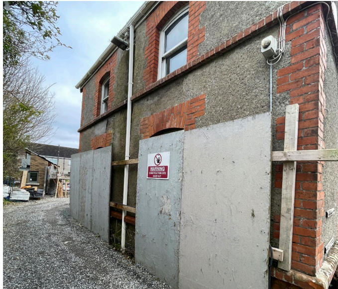
Fig 15: Elevation C. Side access to rear of the site. *Note picture was taken in March 2024 during works to former school-house.
