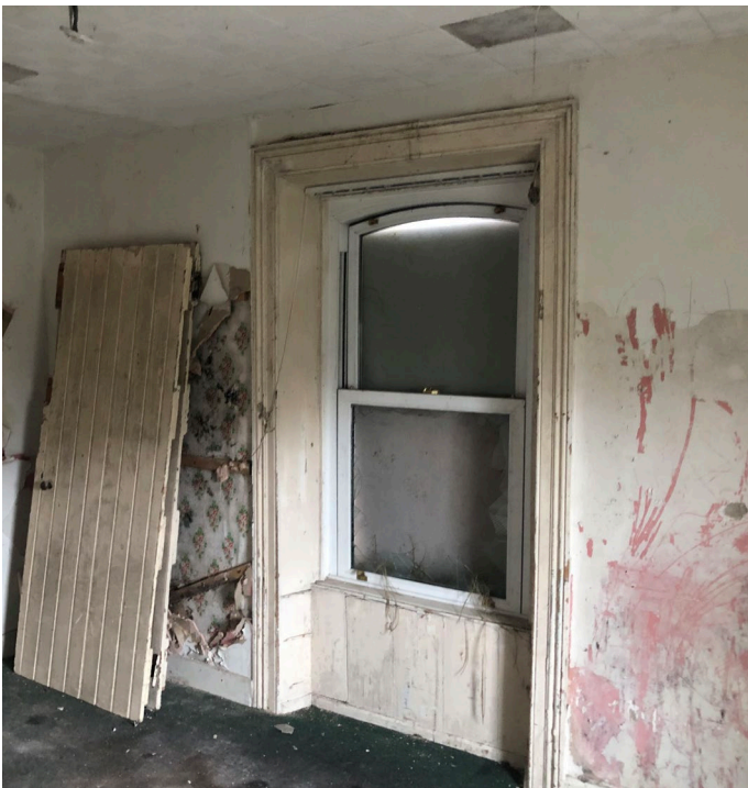
Fig 75: Internal Elevation 11.C. Remains of door. Sash Window and plasterboard have been damaged.
