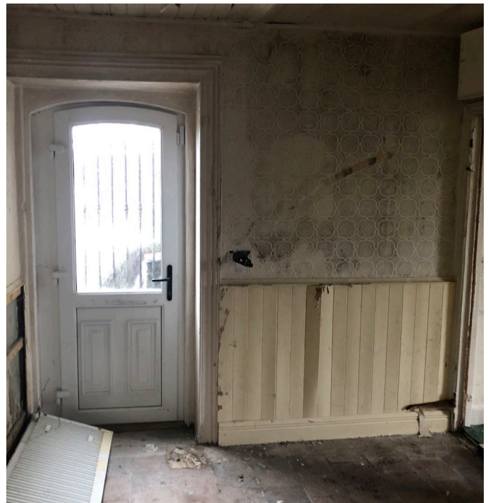
Fig 39: Internal Elevation 3.B. Timber wainscoting panelling has been damaged. Door to rear of the site.
