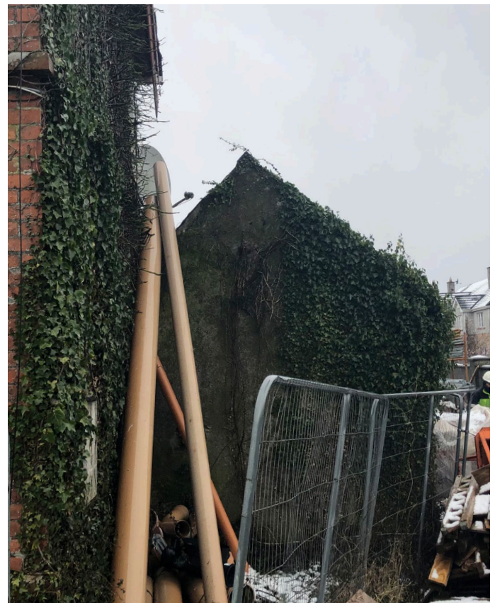
Fig 19: Elevation D extension. Evidence of climbing plants on facade. *Note picture was taken in March 2024 during works to former school-house.
