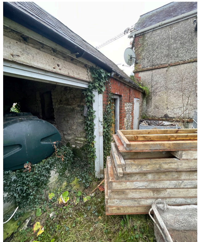
Fig 11: Elevation B extension. Evidence of planting growing in the extension. *Note picture was taken in March 2024 during works to former school-house.
