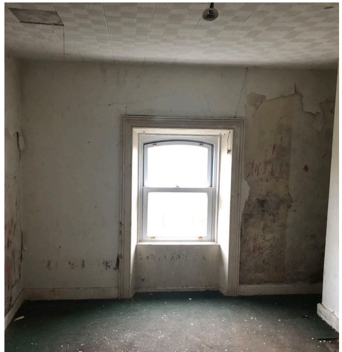
Fig 76: Internal Elevation 11.D. Plasterboard has been damaged.
