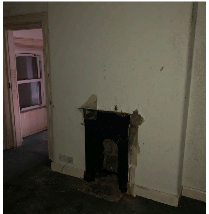
Fig 80: Internal Elevation 12.D. Existing fireplace. Plasterboard damaged.
