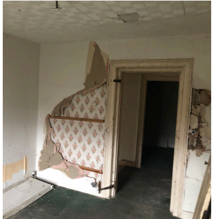
Fig 74: Internal Elevation 11.A. Doorway to room 7. Plasterboard has been damaged.
