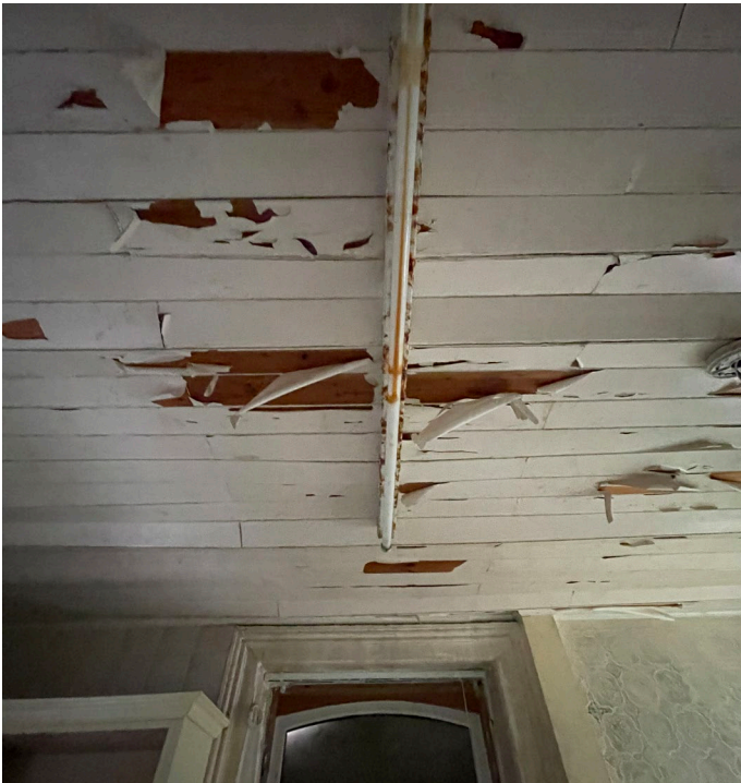
Fig 46: Internal Elevation: False ceiling has been damaged.
