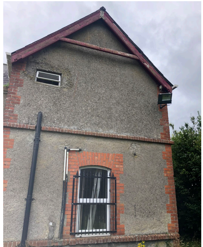
Fig 14: Elevation B. Ground floor window grille fixed to red brick. Existing fascia board has been damaged. *Note picture was taken in July 2020.
