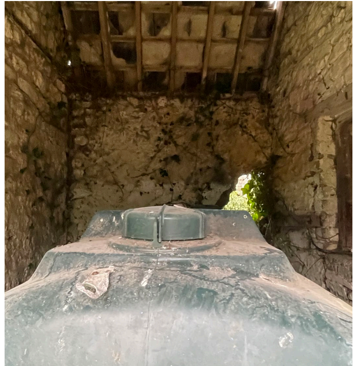
Fig 58: Internal Elevation 6.B. Stone wall has been damaged. Tank stored in room.
