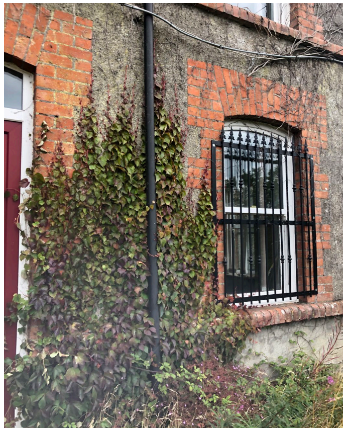
Fig 5: Elevation A. Evidence of climbing plants on front facade. Ground floor window grille fixed to red brick. *Note picture was taken in July 2020.
