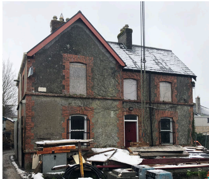
Fig 1: Elevation A. First Floor Sliding Sash Windows boarded up with timber. Evidence of climbing plants. *Note picture was taken in March 2024 during works to former school-house.
