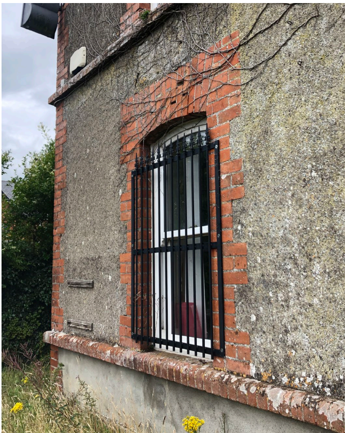
Fig 2: Elevation A Perspective. Ground floor window grille fixed to red brick. *Note picture was taken in July 2020.
