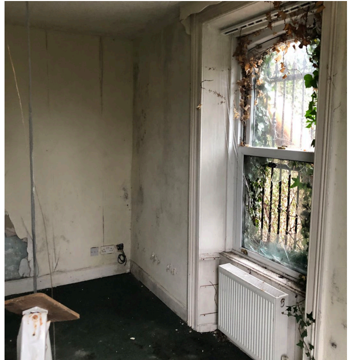
Fig 48: Internal Elevation 4.B. Sash Window has been damaged. Evidence of planting growing into the room.
