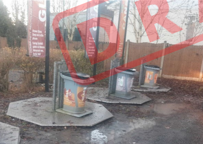
Photo Underground Bring Bank facilities at Ballinahown
