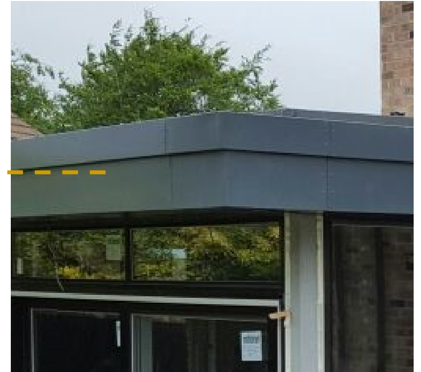
Aluminium close fascia with Single ply membrane to roof of rear extension Elevation
