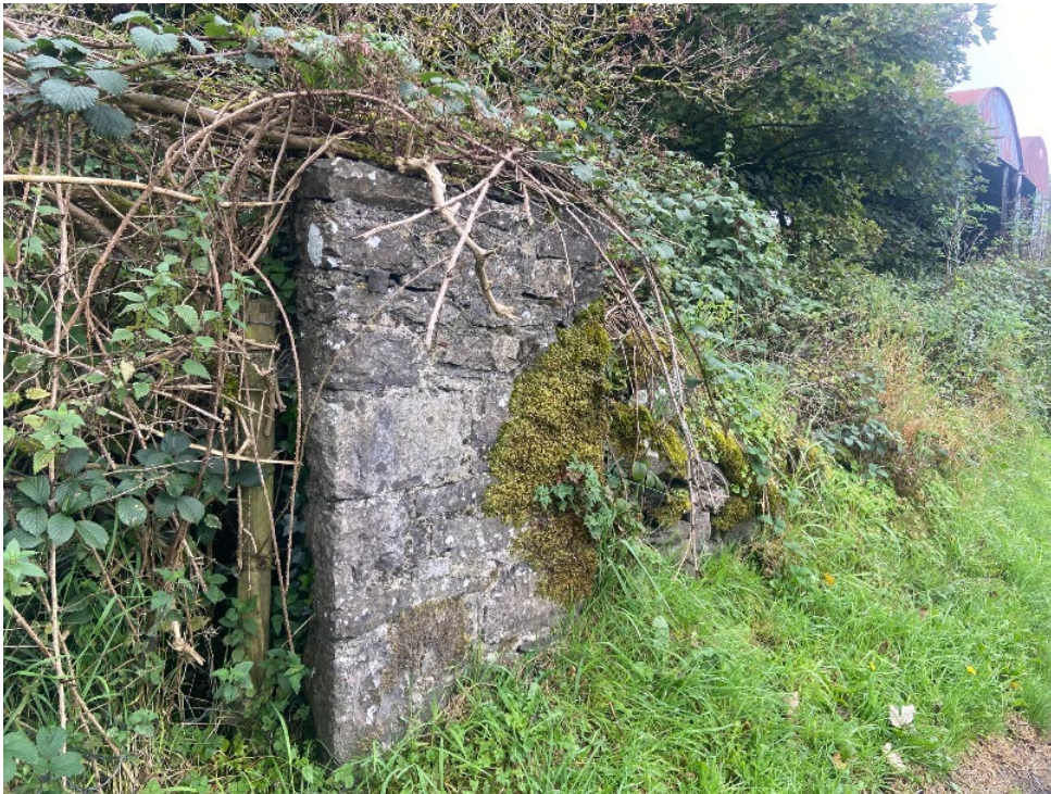
Figure 7: Condition of Historical Wall and potential features to be reinstated.
