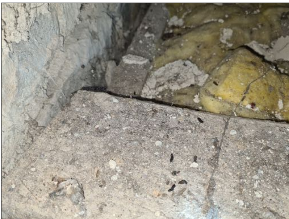
Plate 7. Bat droppings in the attic of the teacher's residence
