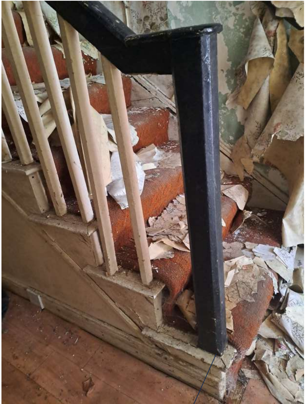
Remedial repair required to secure newel post base
