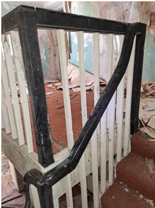
A17: Stairs handrail with gooseneck
