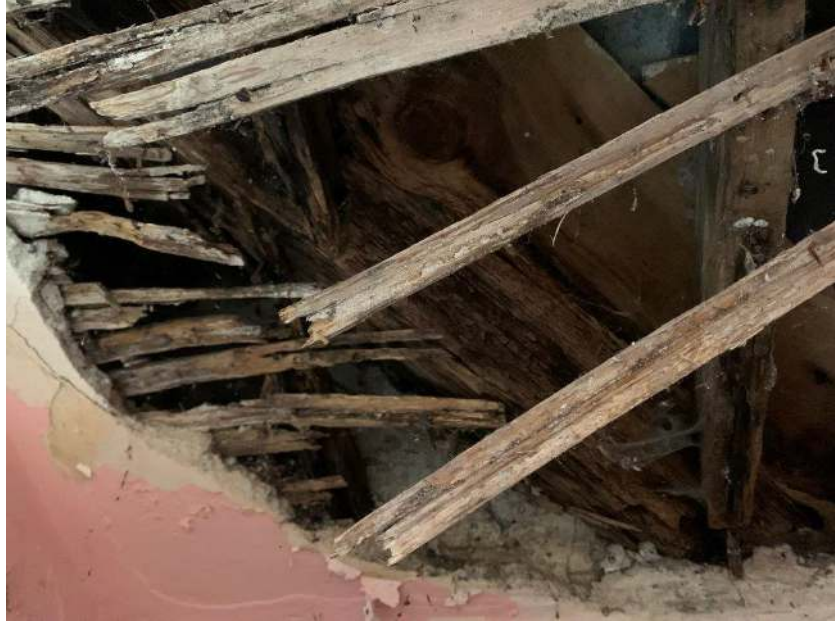
Photo 9 – Valley Rafter Rot
