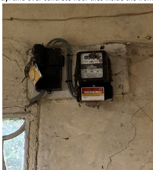
Electrical board. Mounted on timber board.
