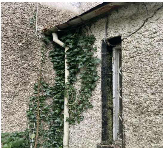
Sample photos of rainwater goods and a toilet flu. These were a mix of PVC and cast iron.
